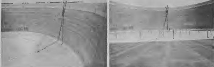
WORKMEN PUT the finishing touches on the gigantic Tank No. 914, the first of its kind at Lago. This huge crude reservoir dwarfs surrounding tanks. TRAHADORNAN TA pone ultimo man na e gigantesco Tanki No. 914, e promer di su clase na Lago. E tanki di crudo grandi aki ta haci e otro tankinan parce miniatura.
